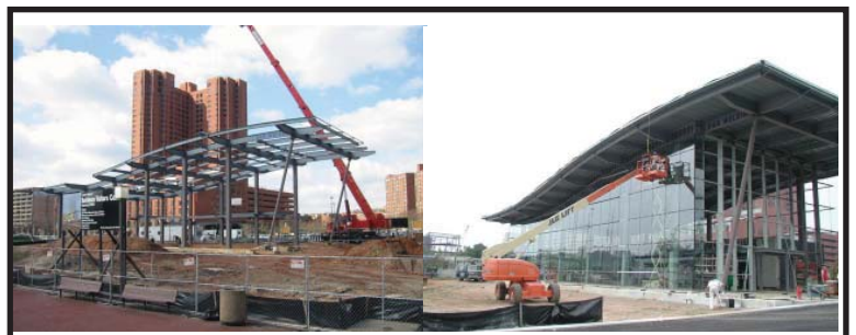
To create the complex wavy roofline of the Baltimore Visitors' Center, B&B fabricated roof beams of tubular steel that fitted into a grid system. To support the cantilevered north end of the roof (the high point in the wave), B&B constructed two sloping ten-inch pipe columns with stainless steel pins. To hold up the main building, they created architecturally exposed 16-inch steel tubes, or columns.
