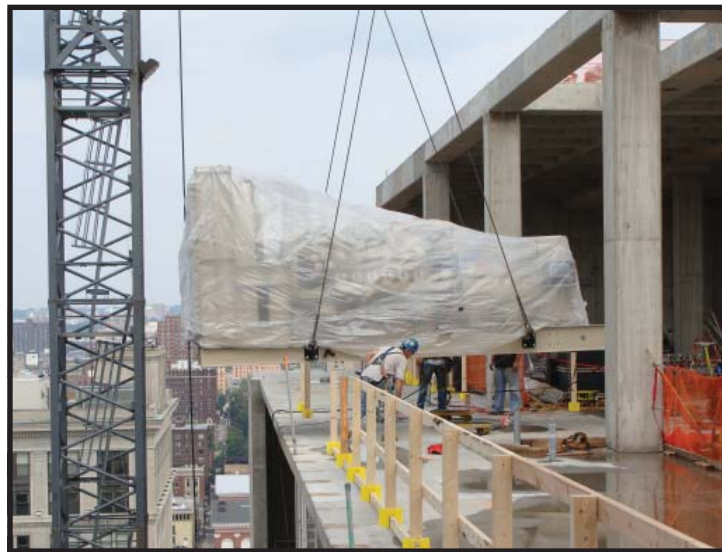
Mercy Hospital, Baltimore, Maryland Curtis Engine provided two 1500 kW MTU Onsite Energy diesel generator sets, ASCO switchgear and eight ASCO transfer switches ranging from 1200 to 2000 amperes. Additionally, Curtis Engine supplied a 600 kVA UPS system from Active Power and a 1500 kW standalone load bank from Avtron Loadbank.
