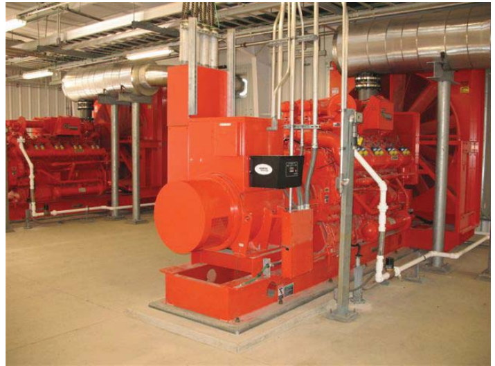
Two WAUKESHA's at Cove Point LNG plant
